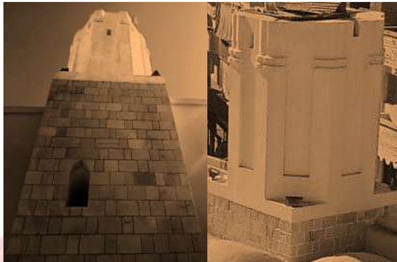
Pl. 7. Two pictures of the minaret after faulty restoration and alteration of monuments by abolishing the transition area between the square and octagonal floors
