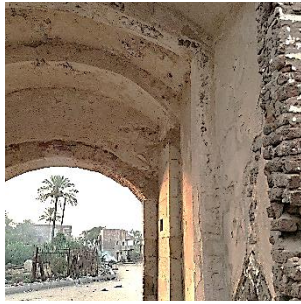
pl. 4. Details of the vault mounted on arches and the vaulted niche to sit the guard on the left side of the gate
