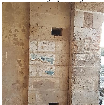
pl. 2. Inputs to place the latch that closes the wooden door of the gate inside
