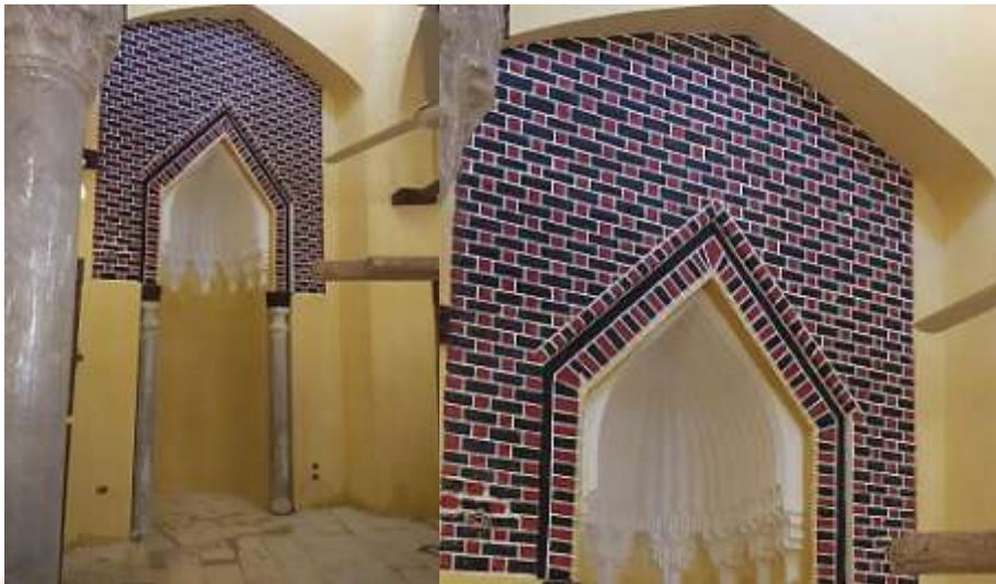
Pl. 2. Two pictures of the mihrab after faulty restoration
