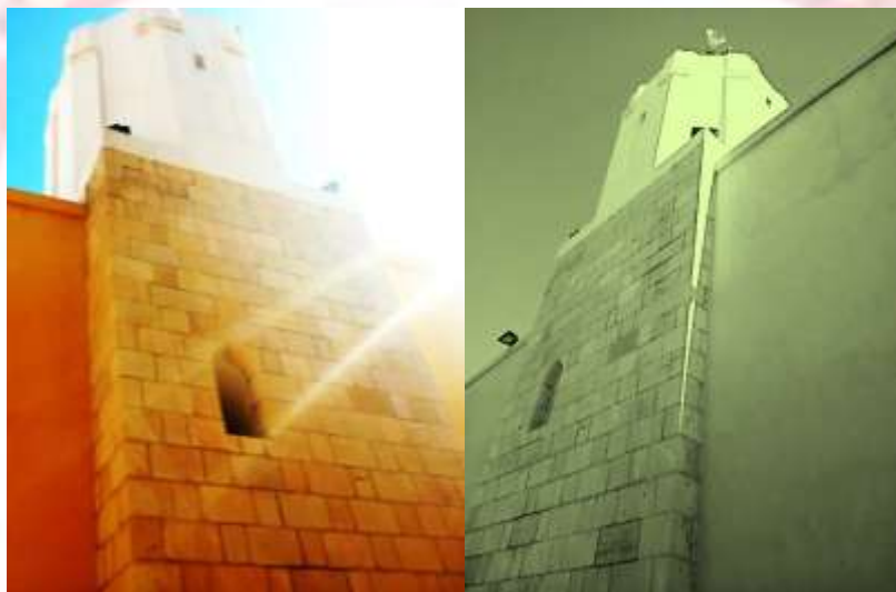
Pl. 6. Two pictures of the minaret after faulty restoration and alteration of monuments by canceling the transition area between the square and octagonal sectors
