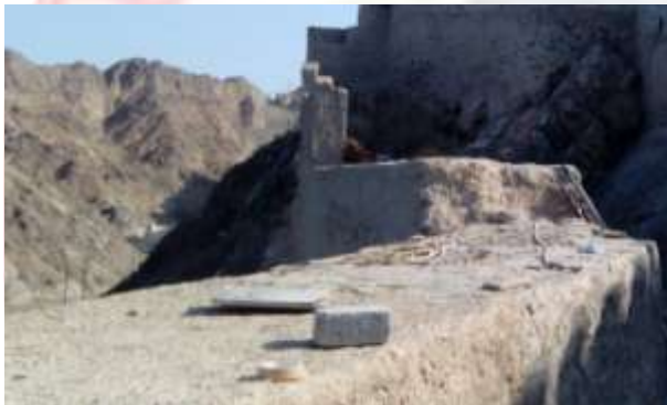
(Fig. 6) The northern wall of the castle and its gradation from east to west (photo by researcher)
