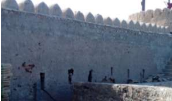
(Fig. 7) The distance between the two towers in the southern wall from the inside (Photo by the researcher)
