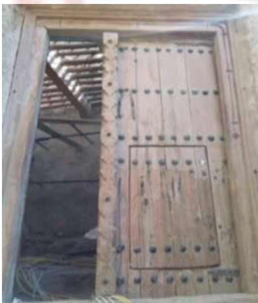
(Fig. 4) The first main entrance located on the southwestern side from the outside (Photo by the researcher)
