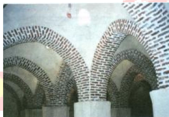
Pl. 18. the pointed arches with two centers that bear the domes in the Church of Anba Shenouda in the Monastery of the Cross
