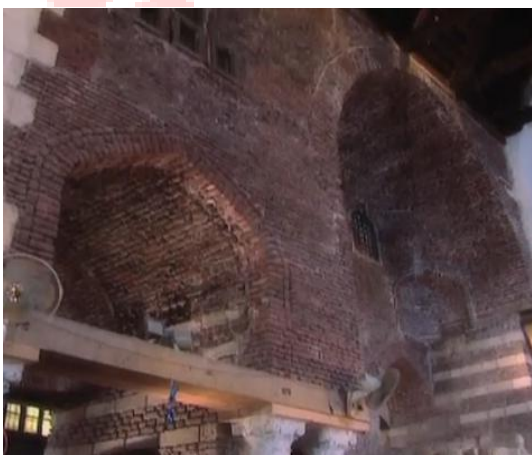
pl. 17. the pointed arches with two centers overlooking the courtyard in the church of Abu Sefein
