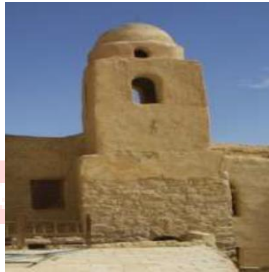
pl. 26. horse shoe arch crowning one of the openings of the bell tower in the Church of Abu Sefein in the Monastery of Anba Paula
